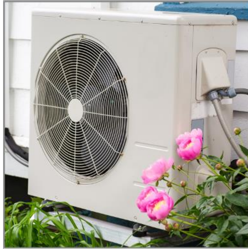
Heat Pump Space Heating & Cooling
